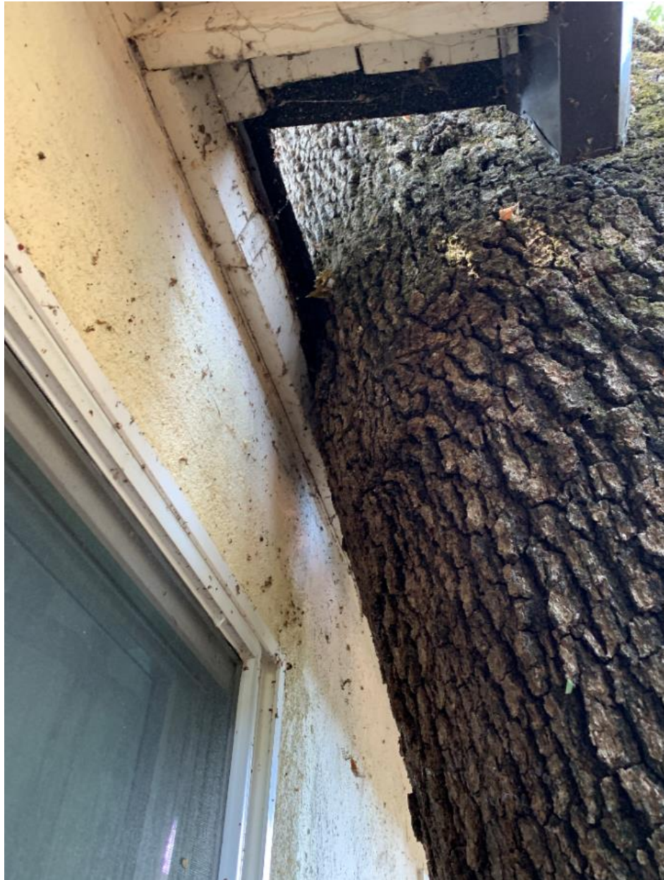
Figure 3. Trunk of Tree 2 in contact with home. Past modifications to the eave visible.
