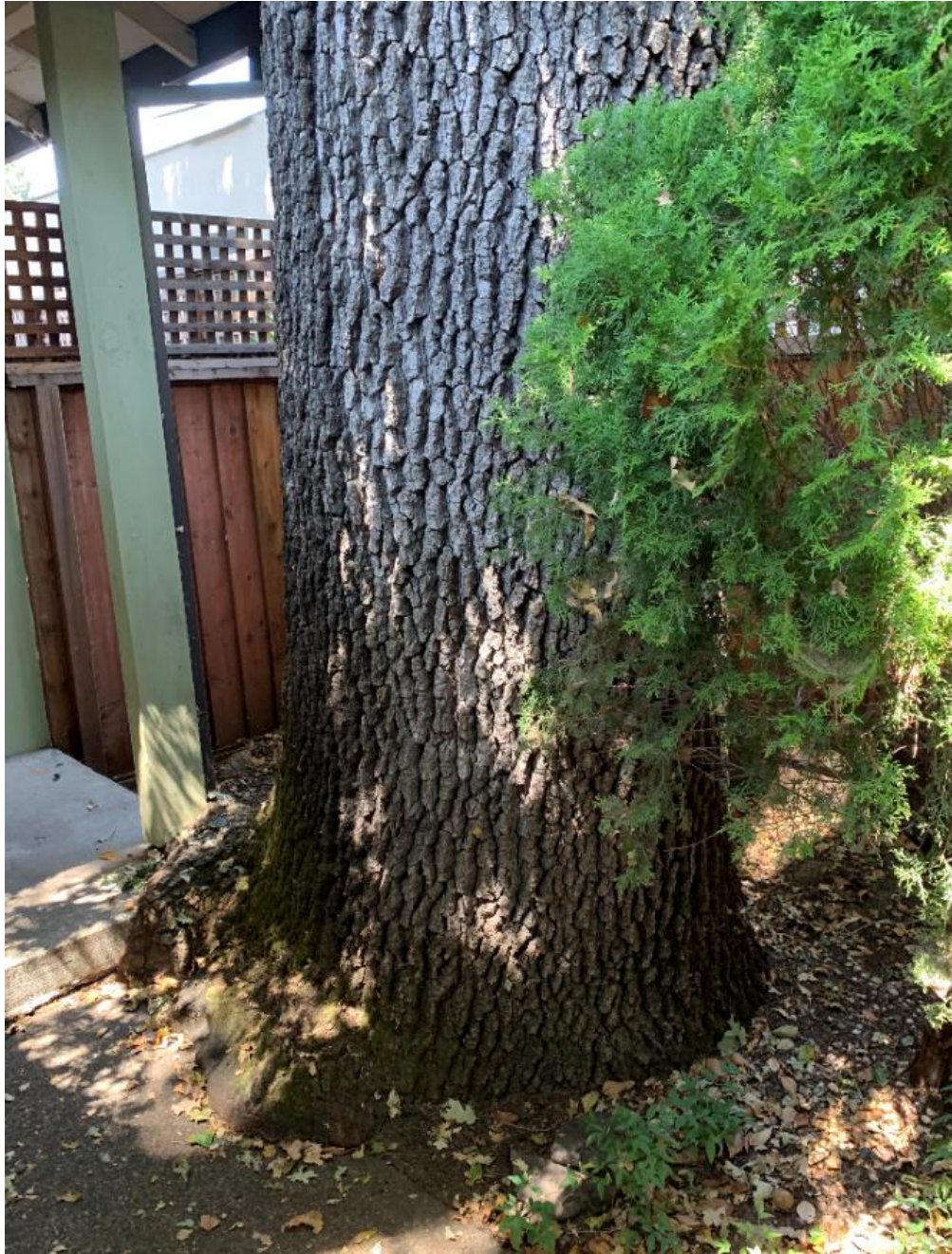
Figure 2. Base of Tree 1 engulfing the sidewalk and stoop.
