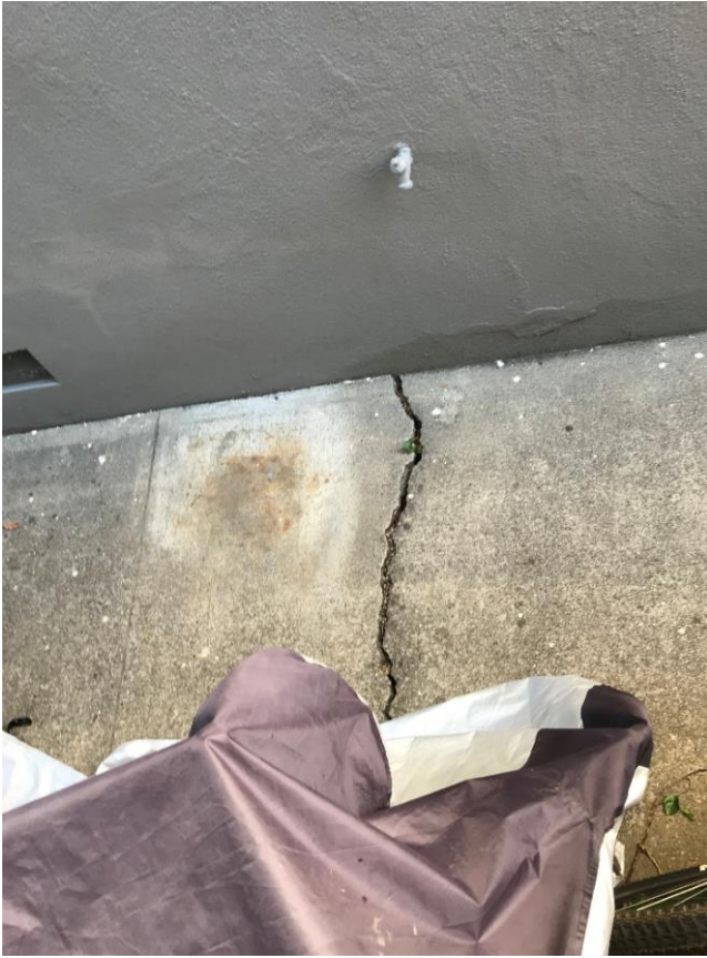
Figure 3. Buckled walkway at 53 Woodland. As viewed from the Nielson property over the fence.
