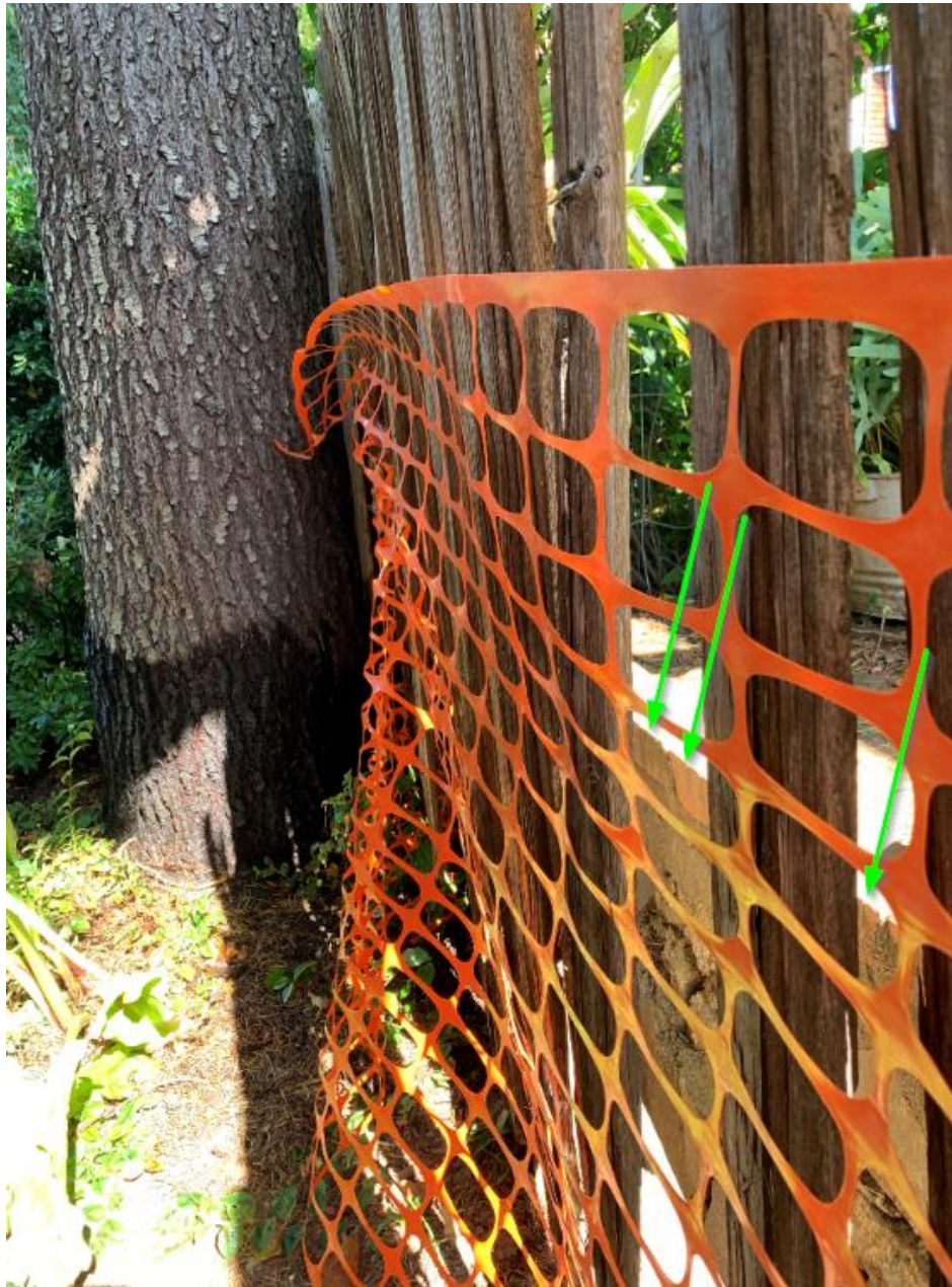
Figure 4. Base of subject tree as viewed from the east-southeast. Top of retaining wall on 19 Cottage indicated with green arrows.
