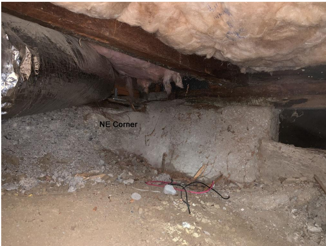
Figure 3 – The tree is within 3.8' of the NE corner of the old foundation and is lifting and breaking it.
