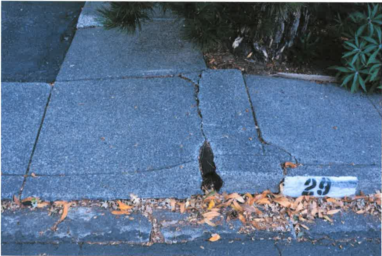
Figure 2 – The uplift of the drainage line has displaced the public sidewalk and curb.
