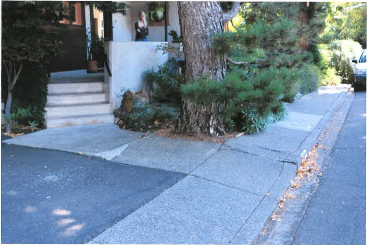
Figure 1 – The subject pine tree is located where it has damaged immediately adjacent infrastructure.
