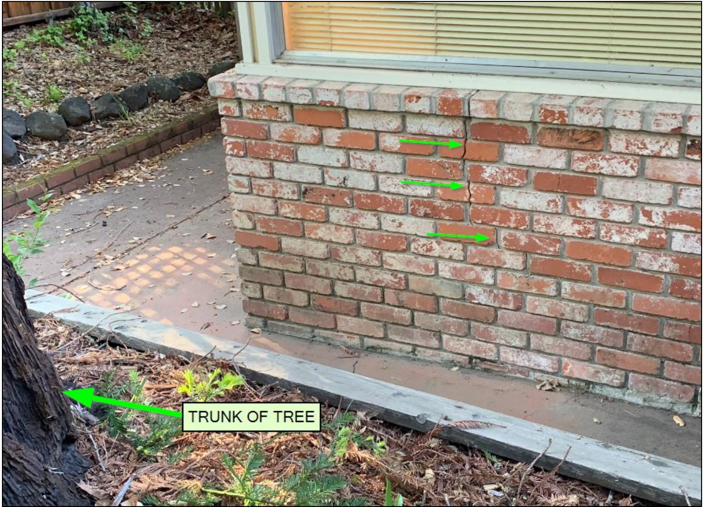
Figure 3. Crack in brick siding
